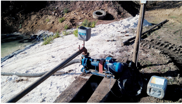
Fig. 3. The pumping station of the washing site of Kaolin Azov LLC, Orikhiv
